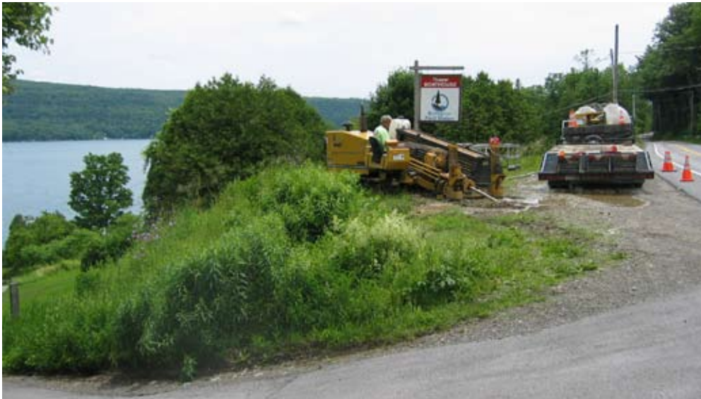
Drilling under Rte. 80 for sewer and telecommunication lines between the Boathouse and Hop House.
